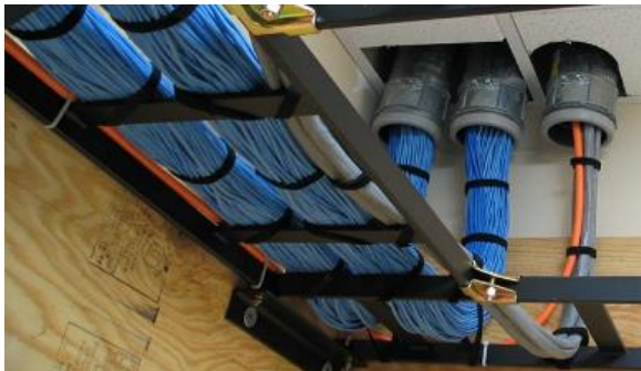
Image: Telecommunications Cabling installed in conduit sleeves and cable tray
