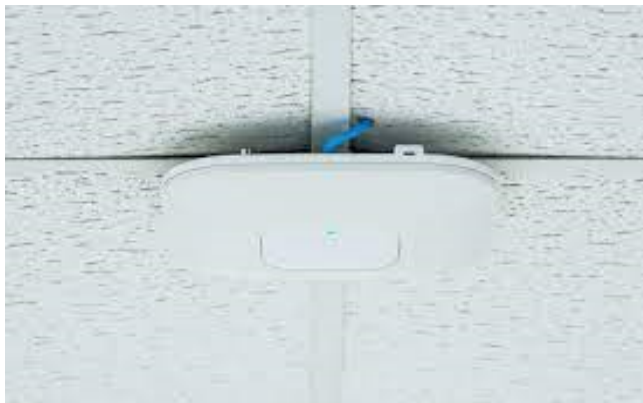
Image: Wireless Access Point mounted to Ceiling
