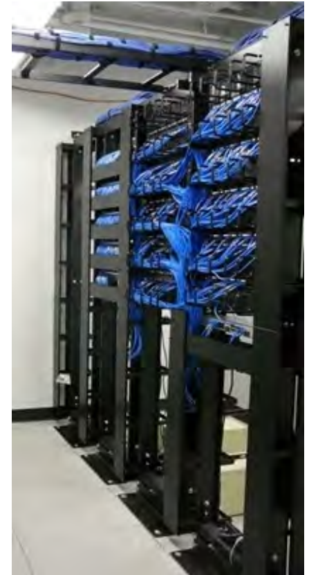
Image: Telecommunications Closet
