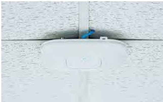
Image: Wireless Access Point mounted to Ceiling
