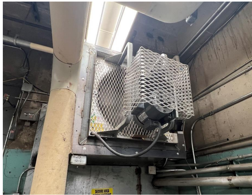
EF-2 Located Within The Mechanical Room
