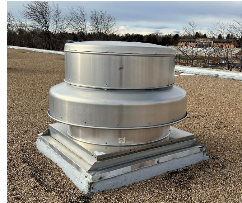
EF-1 Located On Roof
