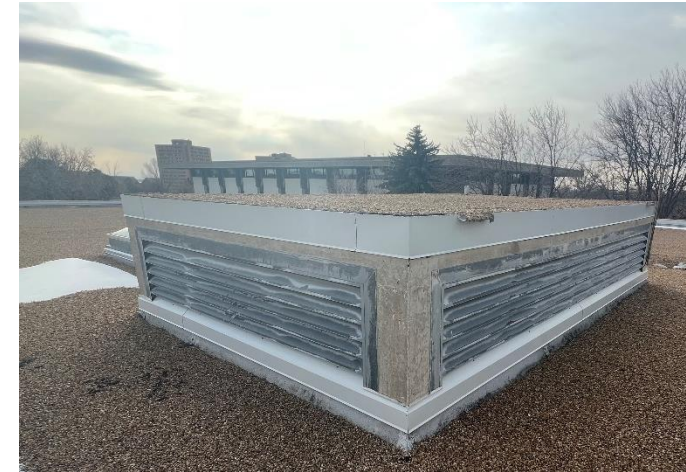
Outside Air Louvers
