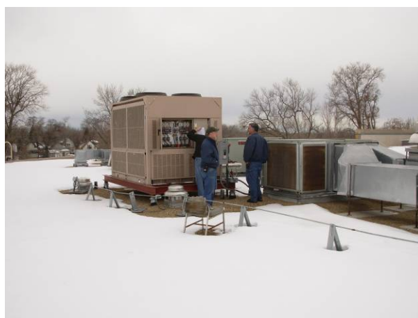
PHOTO – FRASIER HALL CHILLER
