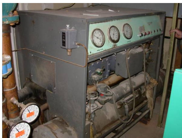
PHOTO – OLD CHILLER AT CARTER HALL
