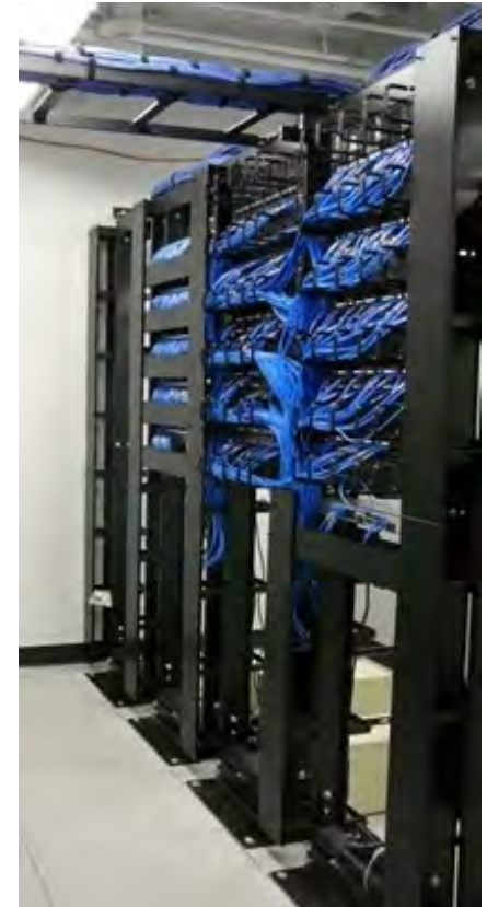
Image: Telecommunications Closet
