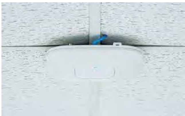
Image: Wireless Access Point mounted to Ceiling
