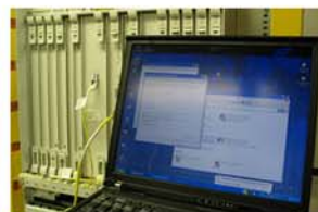
EAp1: Fundamental commissioning of building systems helps save in energy usage.
